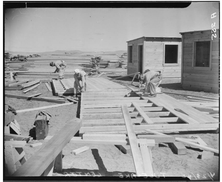
Figure 3: Workers building the first house at Tule Lake Segregation Center, the largest Japanese American Incarceration Camp based in Newell, California. (Credit: Department of the Interior)
