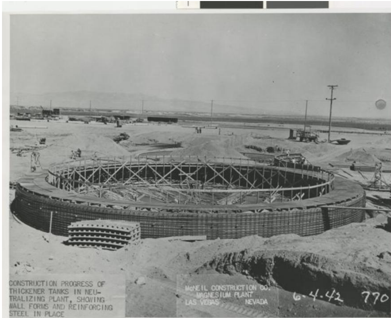
Figure 2: "Construction Progress of Thickener Tanks in Neutralizing Plant, showing wall forms and reinforcing steel in place. McNeil Construction Co. Magnesium Plant." June 4, 1942. (Credit: pho020380, Victor Kunkel Photograph Collection. PH-00072. Special Collections and Archives, University Libraries, University of Nevada, Las Vegas.)
