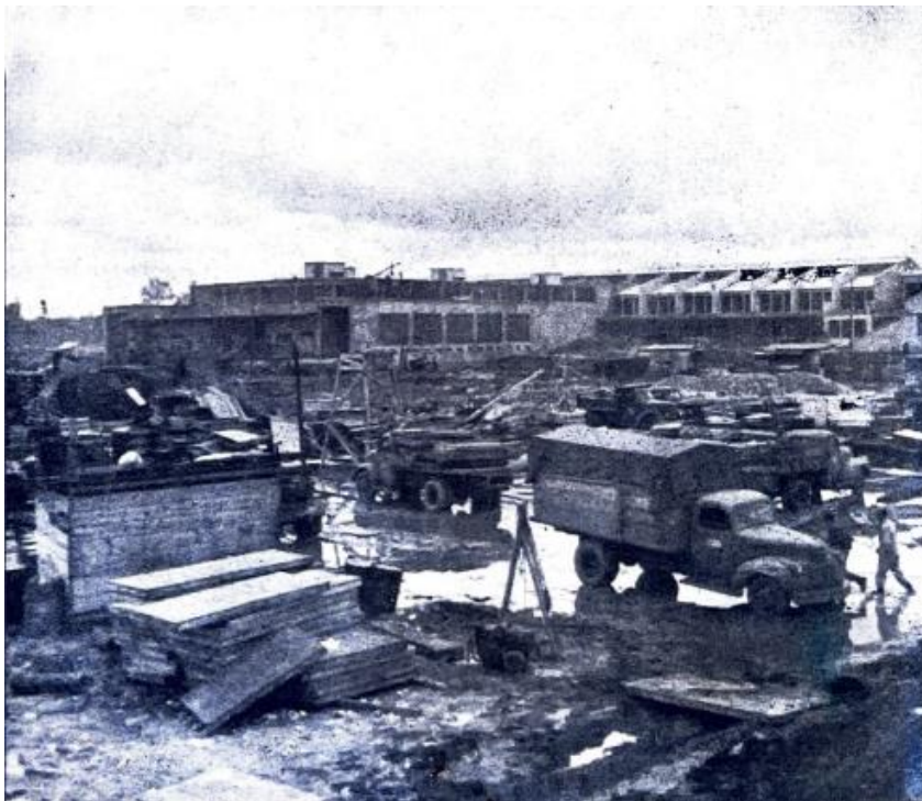
Figure 10: A photo of construction of the Shumaker Naval Ammunition Depot, in a 1950s publication by the depot: "NAD Yesterday and Today." (Courtesy of Public Library of Camden, Ouachita County)
