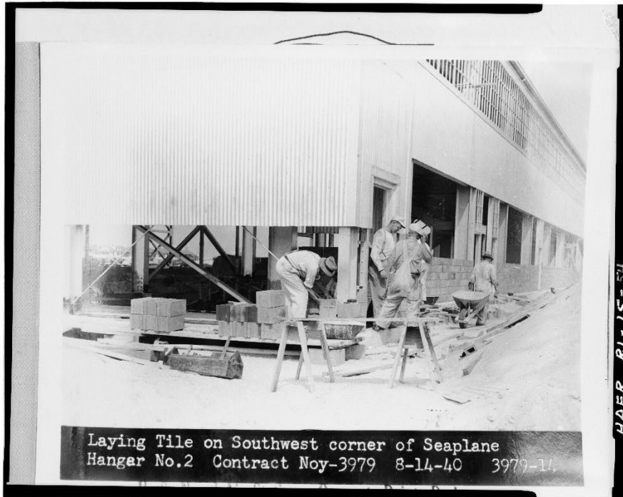
Figure 2: "Laying Tile on Southwest corner of Seaplane Hangar No.2, 8-14-40 (Historic American Engineering Record - Library of Congress)
