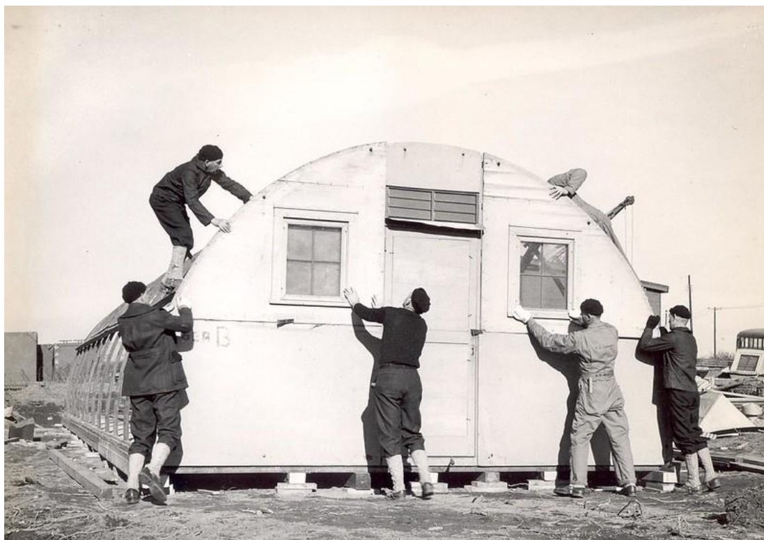
Figure 7: Seabees constructing a Quonset Hut as part of their carpentry training at Camp Endicott in Davisville in 1942. (Courtesy of the United States Navy Seabee Museum Archive)
