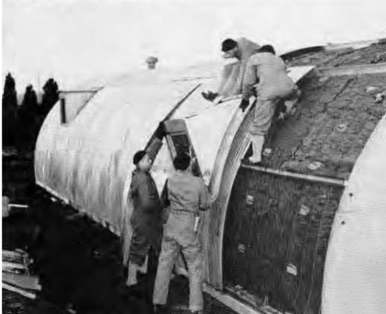
Figure 21: Seabees constructing a Quonset Hut. From a Camp Endicott yearbook by the U.S. Navy Department, Office of Public Relations.
