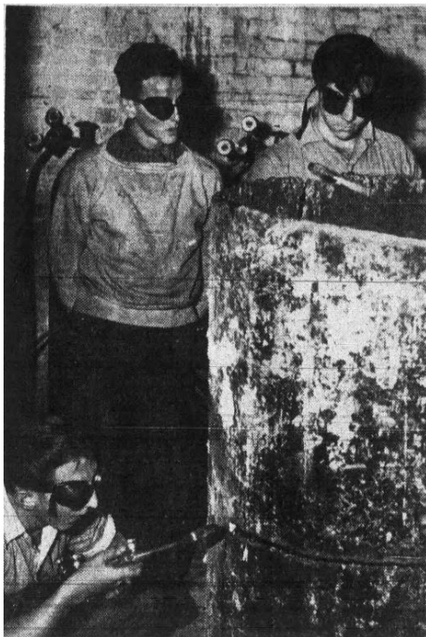
Figure 12: Students training at the Yonkers Work Center of the National Youth Administration aided the city salvage drive by breaking up large objects to make them easier to move to junk yard scrap piles. Here three men were cutting apart a boiler. ( The Herald Statesman , October 3, 1942)
