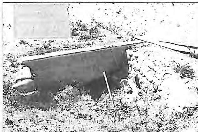
Figure 3. Photograph of RF 1, a cobbles-lined concrete culvert, facing south. This feature was initially documented in the previous Class III survey (Jones 2009).
