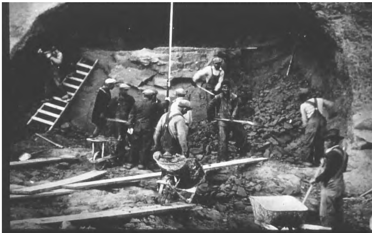
Fig. 1: Workers excavate one of the Summit Road tunnels during New Deal-era construction. Courtesy Scotts Bluff National Monument Archives.
